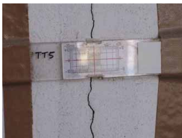
Monitoring a crack on a column in Former Marine Police Headquarter, Hong Kong Source: S. S. Imon
